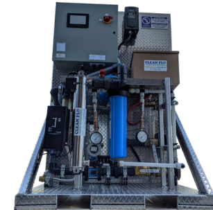
Treatment and Control Systems
