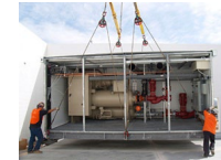
Modular Central Plant
